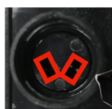
V Pin Transformer PD12 65446
